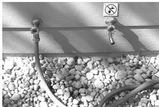
On-site water reuse systems that allow graywater to be used for outside irrigation require a separate hose bib clearly marked for non-potable use only.
